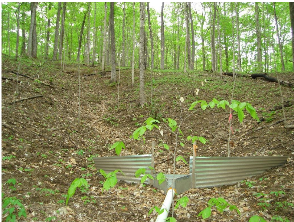
Photograph 5-3. Photo shows how corrugated metal sheets were buried to divert overland flow into the flume.
