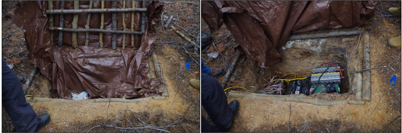
Figure 7-15: Subterranean power source composed of log frame and hatch wrapped in tarp containing three Everlast batteries wired together and attached to inverter and a solar box. Two solar panels were subsequently located six meters upslope.
