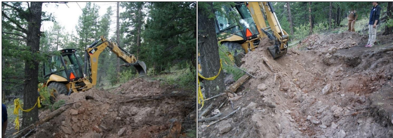
Figure 7-21: Left - Backhoe negotiating the steep landscape after requested by anthropologists to excavate the difficult terrain. Right - excavation of what would expand to a 5m x 5m exhumation site. Note size and density of granite occlusions.
