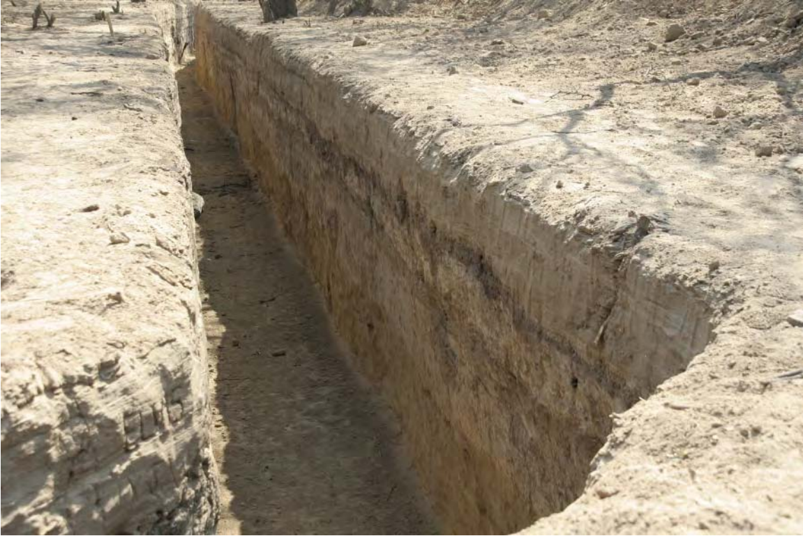
Figure 8.5. The profile of a new drainage channel under construction at the Great Plaza.
