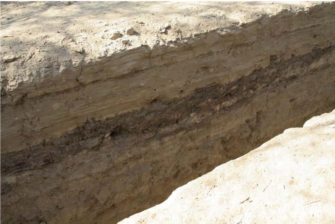
Figure 8.6. The profile of a new drainage channel under construction at the Great Plaza.
