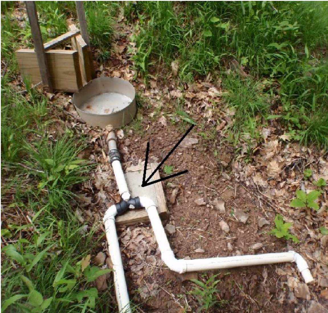
Figure 9. A splitter (see arrow) installed on section 7, to prevent tank overflows. Splitters were also installed on sections 3, 4, and 6. Approximately one-half of the flow through the pan was delivered to the tank (left PVC pipe in this figure) and the other half was diverted onto the forest floor (right PVC pipe in this figure).
