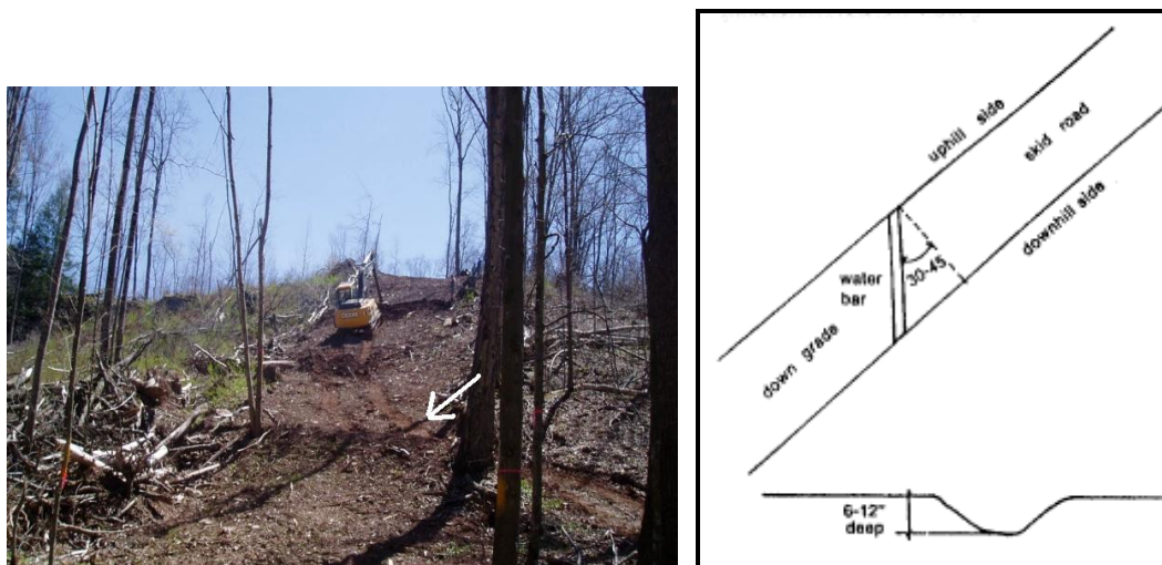
Figure 2. A water bar installed in the field following pipeline installation, and a schematic of a water bar installed on a skid road following WV silvicultural BMPs (WV Division of Forestry, 2005). The method shown for the skid roads is essentially what was used for the pipeline.
