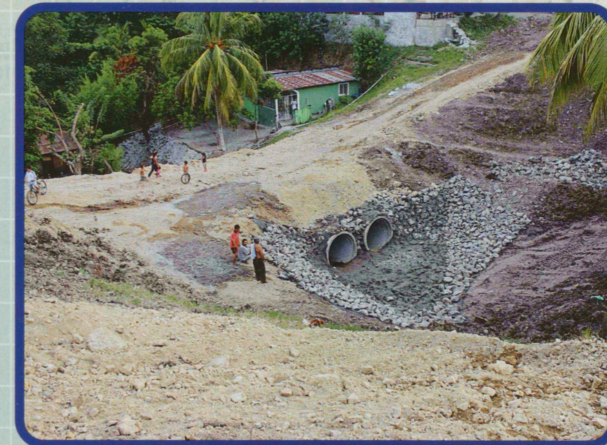
Pimienta residents make use of their newly completed bridge, which opened the town back up to neighbouring communities after 13 years.
