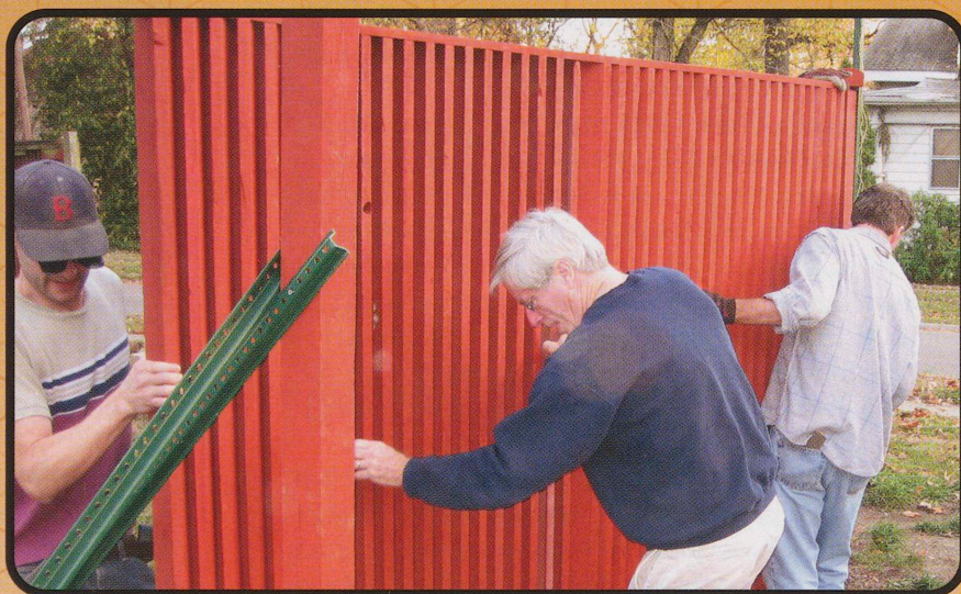
Larry Weatherford (center), and other volunteers on the RBF Dome NFP board, are shown taking part in the ongoing work to restore the unique, Fuller-designed fence that encompasses the dome.
