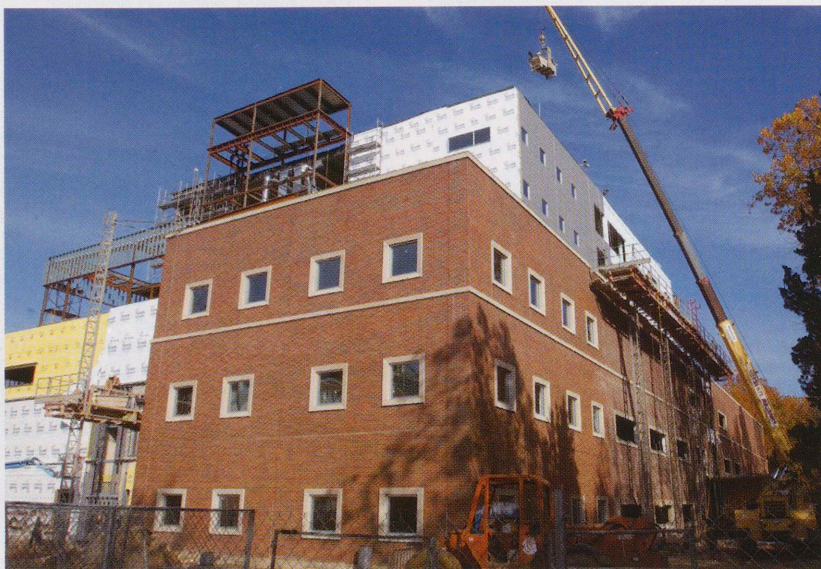
The project includes a complete refurbishment of the existing building and a 50,000-square-foot addition.
