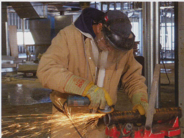
David Crews of Murphysboro smooths the edges of a torch-cut pipe that will be a leg for a new cooling tower on the roof of Morris Library at Southern Illinois University Carbondale.
