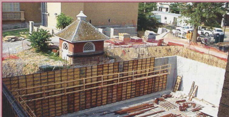
Viewed from the second floor, the foundation and basement of the 20,000 square foot addition is displayed on the west side of the building.
