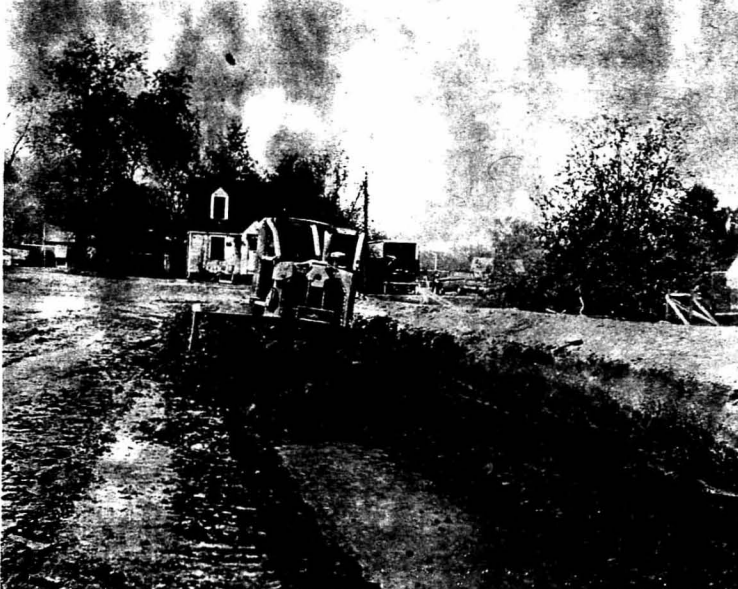
COMMUNICATIONS GROUNDWORK - Giant earth moving equipment is already busy cutting away slices of land to make way for the new School of Communications building in the Chautauqua area. The $3,080,721 structure will be built in two phases and will provide space for the Speech, Speech Correction, Theater and Radio-Television departments. The second phase will house the Journalism, Printing and Photography departments and Film Production Service.
