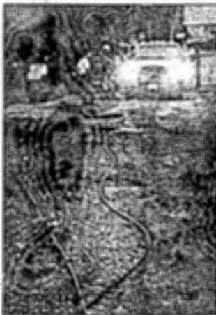
Workers from the utility company CPS such around McDaniel Street near Oakland to assess the damages that occurred when a tree landed on the streets power lines. As of press time power was still out on the block.
