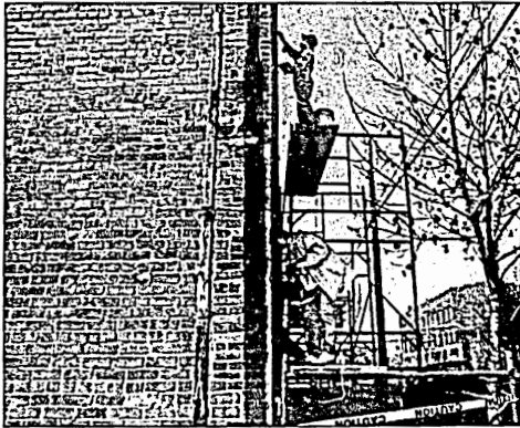
Debbie Gregory, of Murphysboro, and husband Rick tuckpoint a building on Route 13 headed West Monday morning. The Gregorys work for Shannon Waterproofing in Murphysboro. RONDA YEAGER DAILY EGYPTIAN
