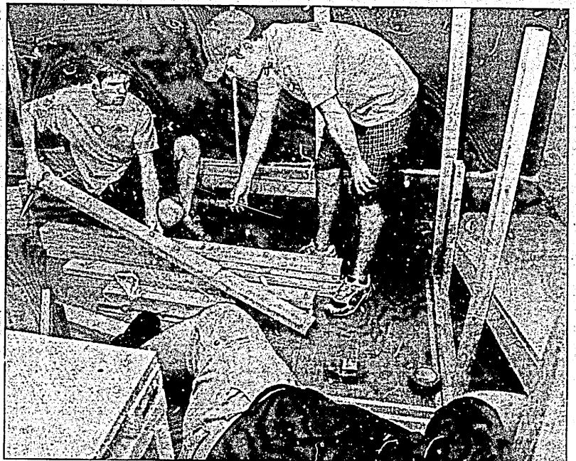
ROMA YEAGER - DAILY EGYPTIAN Andy Bradbury (clockwise, top left), Mike Quick and Jeff Russell work with two-by-fours to build the structure of their haunted house in Wright II Thursday evening. The group of 20 some students are putting on a haunted house from 6 to 8 p.m. tonight, Tuesday and Wednesday nights in the basement of Wright II in University Park.
