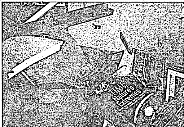
Debris fills the living room of the home of Robert Daniels, a senior studying mining engineering, Wednesday after a line of storms passed through southern Illinois late Tuesday. PHOTO BY PAT SUTPHIN
