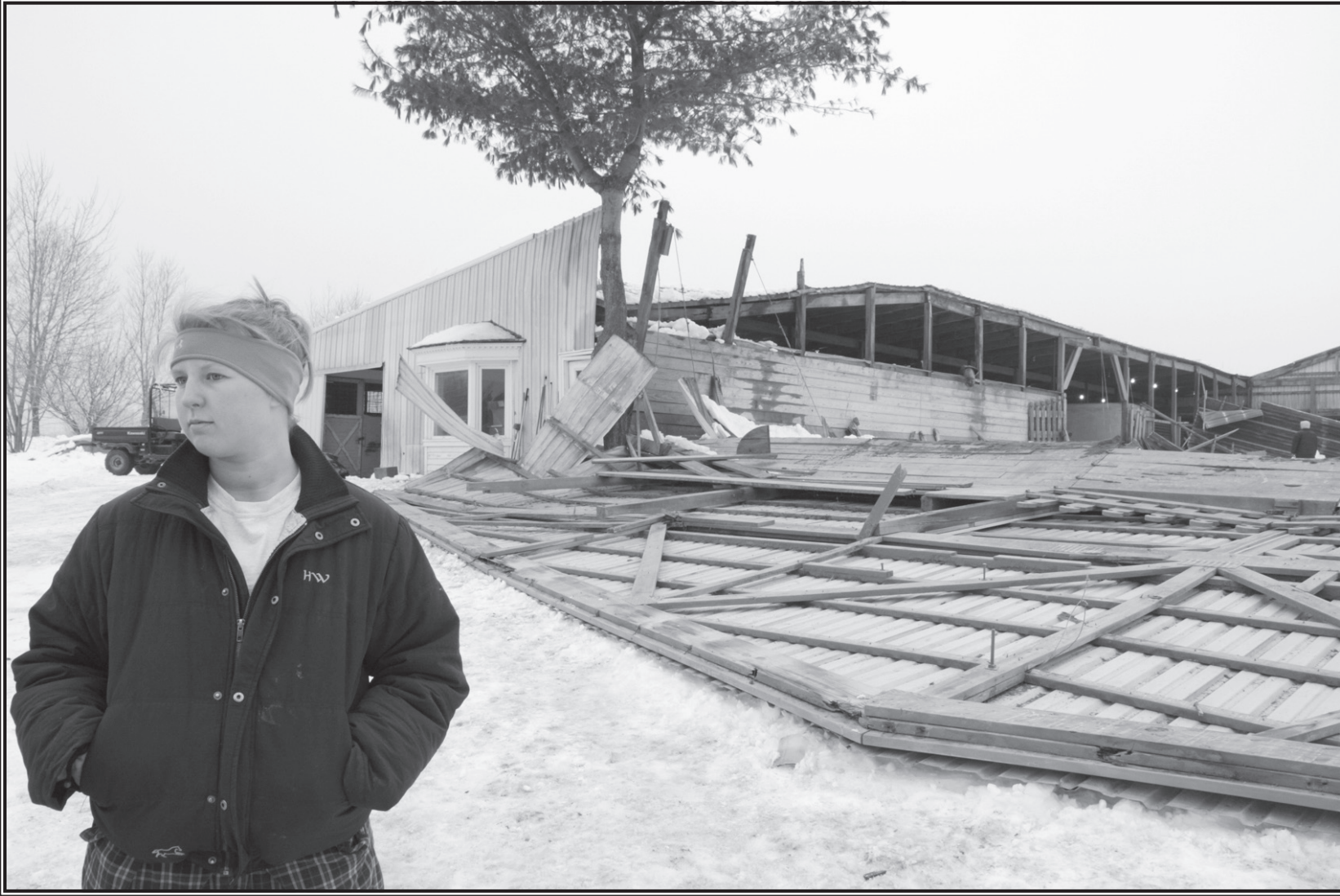
Courtney Carson, of Anna, stands in front of what remains of Le Cheval De Boskydell boarding stables after this week's storms caused the 40-year-old barn to collapse. "We have to rebuild. This is our life. This is how we make our living. It has to go back up," stable owner Jill O'Donoghue said.
