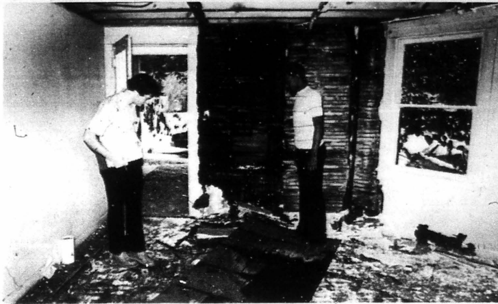
Stan Frazer, to the left, and Horace Pierson, Carbondale Code Enforcement officers, re-inspect a house at 301 S. Logan which was in violation of the housing code. The house is being torn down, because it is economically unfeasible to repair it. (Staff photo by Daryl D. Littlefield)
