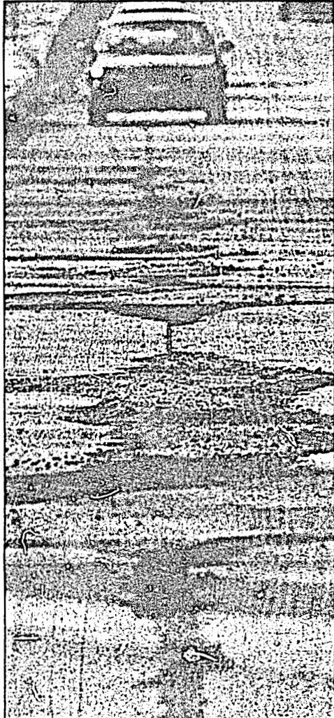
ISAAC SMITH | DAILY EGYPTIAN Evering commuters face pothole damage Friday on Chautauqua Street in Carbondale. City Manager Alan Gill said road crews have put down more salt than usual this season, which has exacerbated the city's pothole problem.
