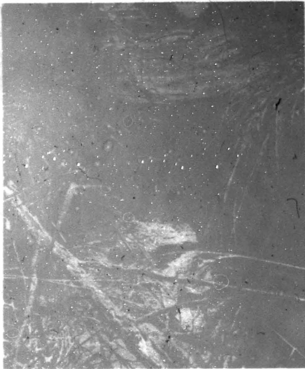
This caved-in asphalt drainage ditch at the northwest corner of the IGA parking lot has had extensive erosion.
