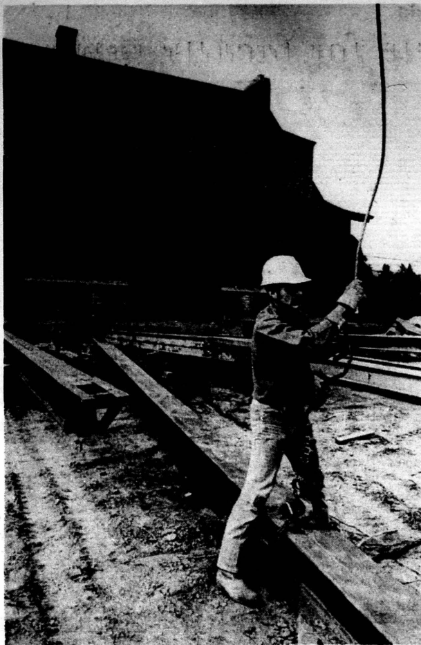
Charles Coleman, an employe of Cruickshank House Moving of East St. Louis, guides a beam under the house at 215 W. Elm St. The house is being moved to a location on University Avenue by its new owner, Henry Fisher. (Staff photo by Peter Zimmerman)
