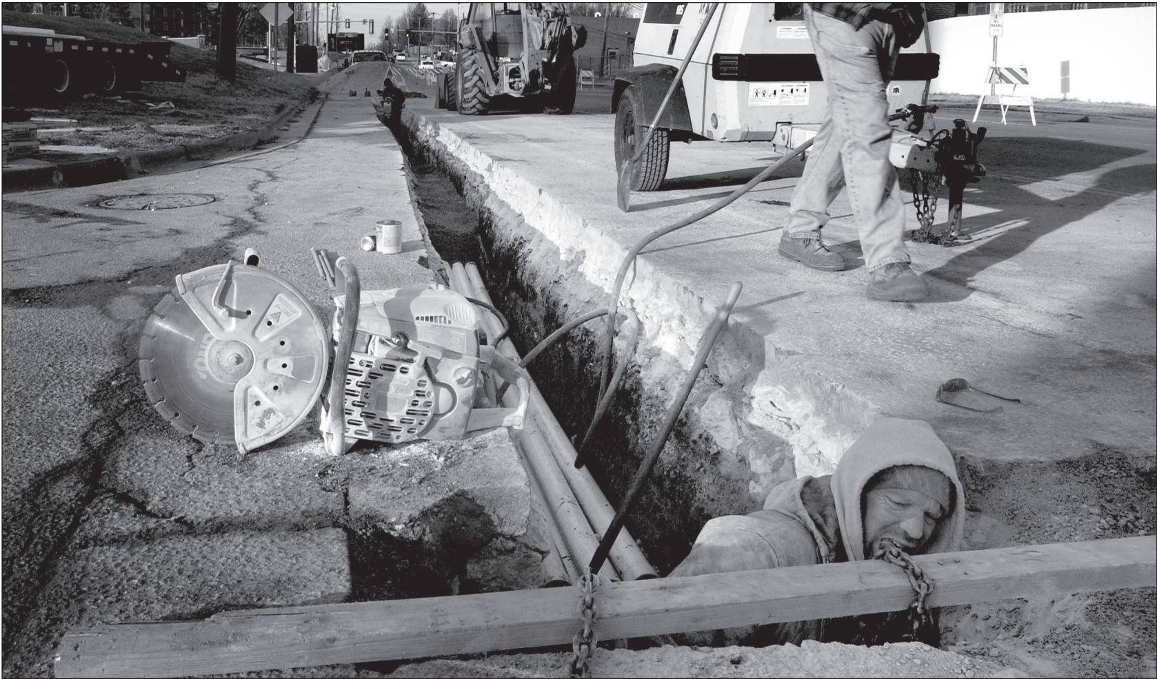
Matt Nollman works to lay fiber optic cable Tuesday evening for Verizon on Wall Street. Nollman said the work will continue for the next couple of days.
