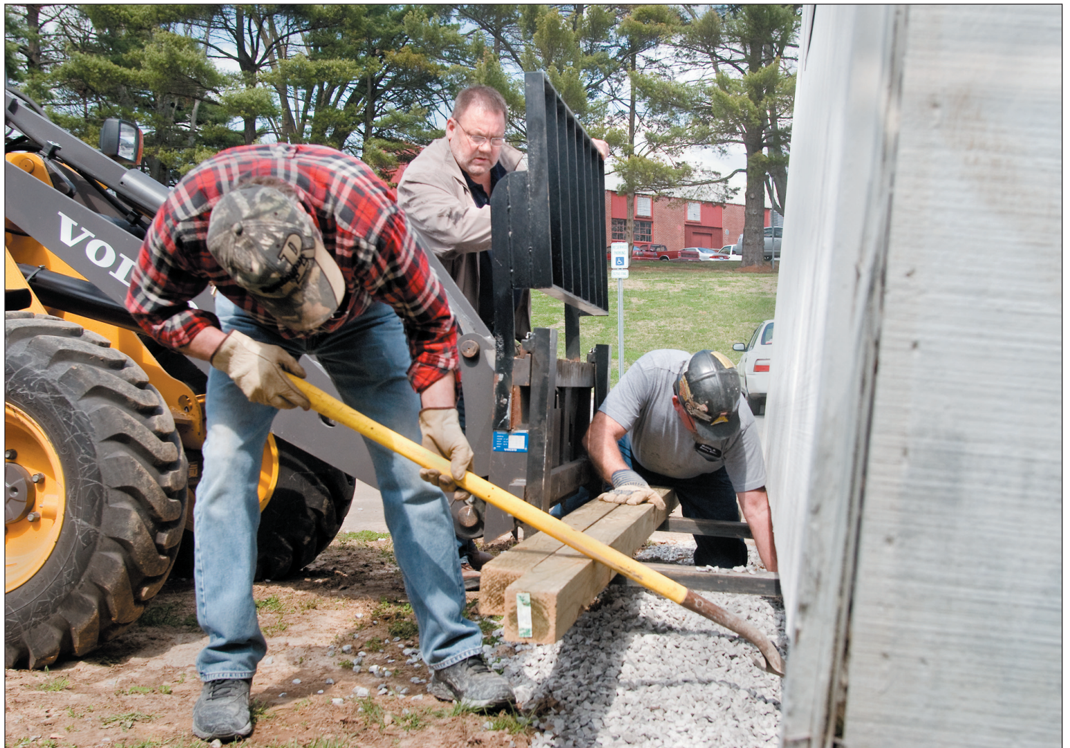
BRANDON CHAPPLE | DAILY EGYPTIAN Mark Goetting, center, a construction manager for SIUC, directs John Spence, left, and Steve Parry while they remove excess rock from underneath the SIUC tennis shed near the tennis courts Monday. The shed was moved to accommodate the Saluki Way construction effort. Workers have begun initial work on the new football stadium, which is expected to be ready by the 2010 season.
