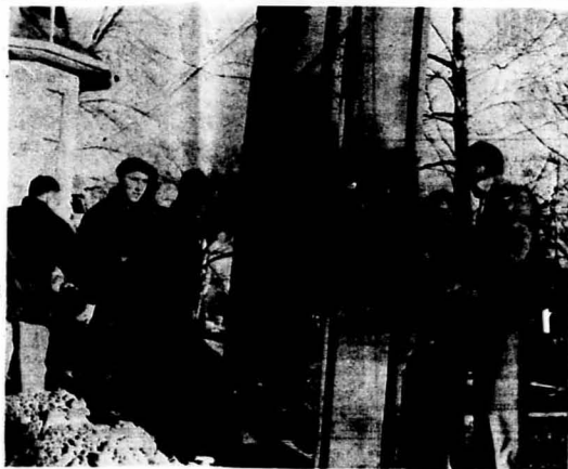
THE FRAMEWORK for a campus marquee being put in place on the corner of Grand and University, across from the main gates. The SIU signboard is being donated to the University by Theta Xi fraternity from proceeds of last year's Variety Show. It was designed by the SIU Architectural Service and will cost approximately $750.
