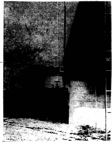
REFILLING A workman refills the storage tank at the Chatauqua Housing Project with propane gas which the mixture had been drained out.
