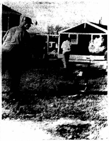
TRICKY BUSINESS A workman shies away from the open jet which has just ignited to burn off the gas which nearly caused a disaster at the Chatauqua Housing Project Saturday. Gas was piped from the buildings and burned before it could explode.
