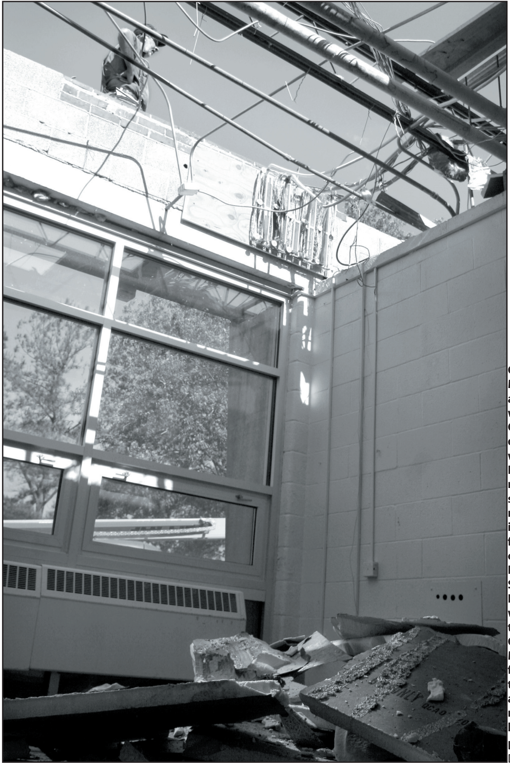
Gary McGowan, a carpenter with J & L Construction, directs other workers on Lewis School's roof while standing near a hole in one of the fourth-grade classrooms Friday. Students from Lewis School will attend the adjacent Carbondale Middle School for the rest of the school year as workers repair the building.
