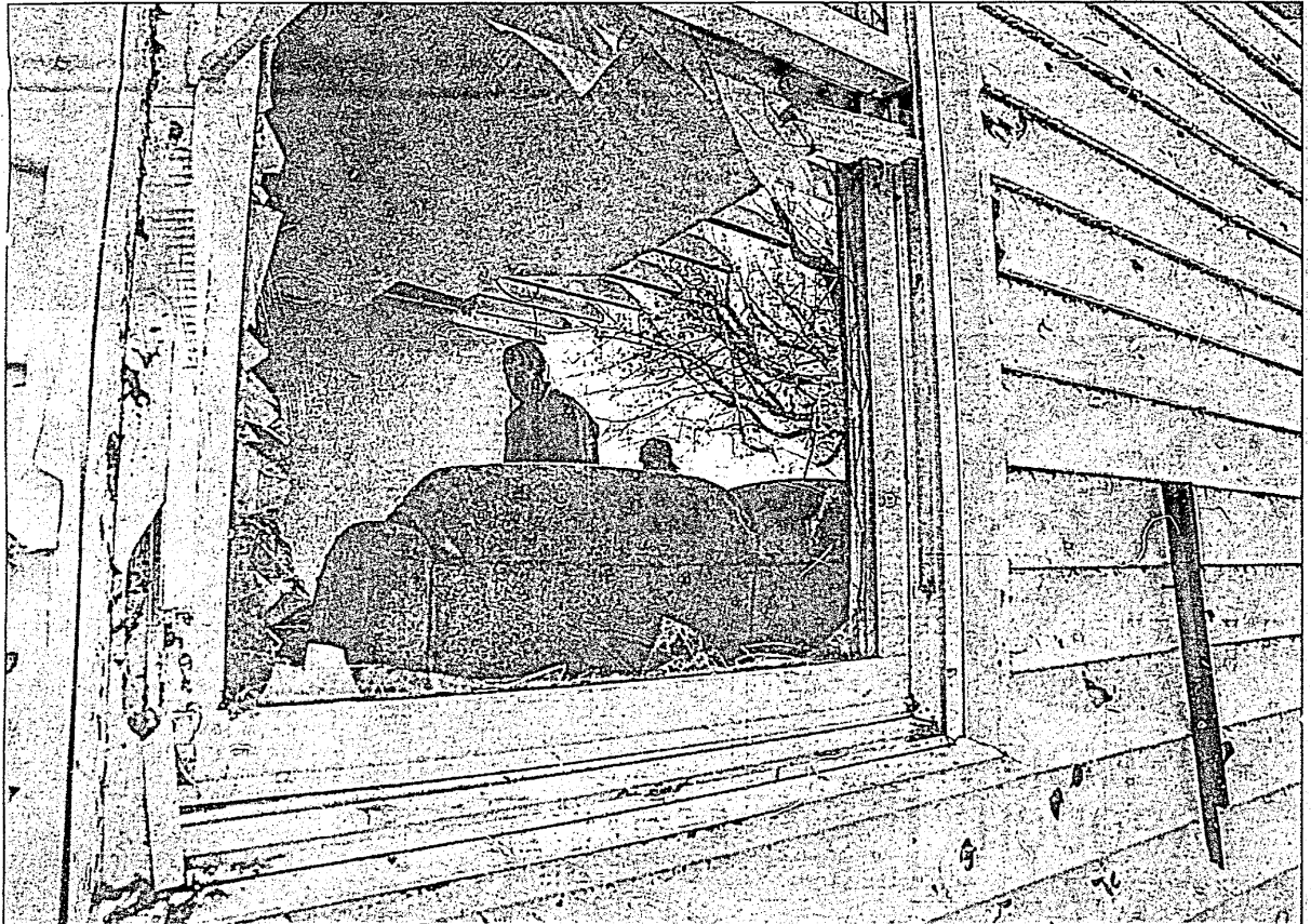
Volunteers help move salvaged items out of Billy and Doris Robertson's house. The front of the Robertson's house was completely torn off during the tornado that hit Fairfield and Sims on April 21.
