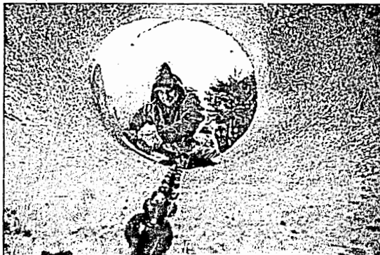
Don Simpson of Mid America Services secures an old drainage pipe to a flatbed trailer near the current construction of the Mill Street underpass in downtown Carbondale.
