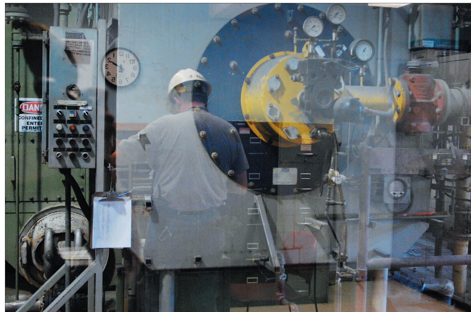
ABOVE: The package boiler was installed in 1990 and is used during emergencies only because it quickly creates steam that can be used for heating or cooling buildings. It costs six times more than the main boiler, so it is used sparingly.
