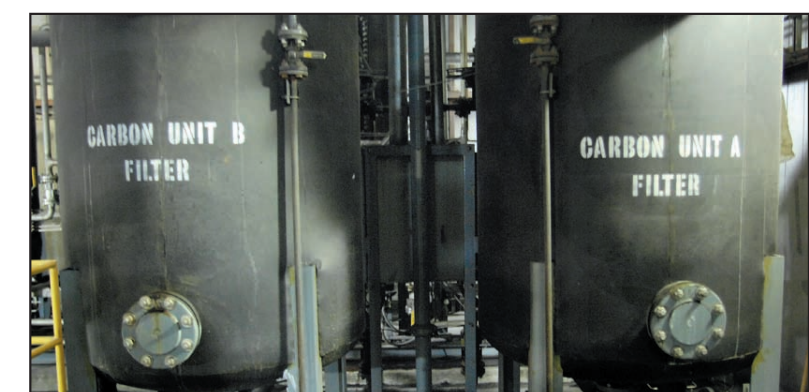
Carbon filters are used to remove minerals, such as chlorine, from water in order to purify it for the boiler. It is part of the de-mineralizer system. Impure water would create mineral buildup in the boiler tubes and reduce efficiency.
