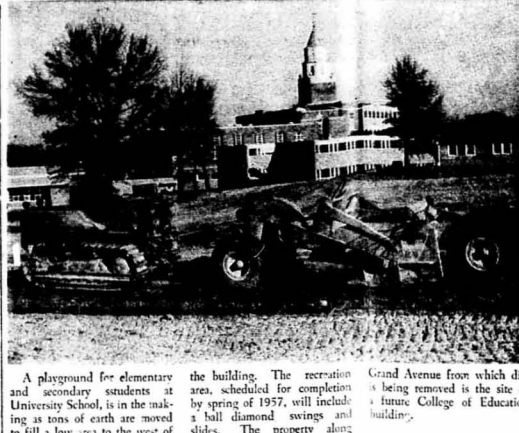
A playground for elementary and secondary students at University School, is in the making as tons of earth are moved to fill a low area to the west of the building. The recreation area, scheduled for completion by spring of 1957, will include a ball diamond swings and slides. The property along Grand Avenue from which dirt is being removed is the site of a future College of Education building.
