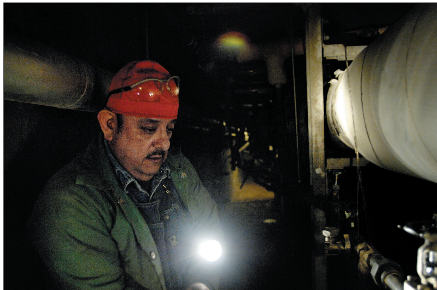
ABOVE RIGHT: Missing and water-damaged ceiling tiles are common in Faner Hall due to its leaking roof. BELOW RIGHT: Rudy Amaro, a university pipe fitter welder for nearly 14 years, said there are many deferred maintenance areas in the campus's underground tunnel system.
