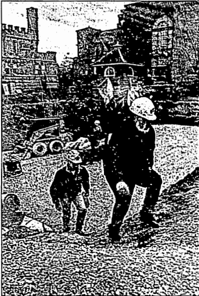
Herold Hennis (front right), project superintendent from Streator, and Josh Sayer (left), of Holcomb Engineering from Carbondale, emerge from the deep ditch dug behind Altgeld Hall on Wednesday. The ditch is the start of a foundation for the Altgeld extension, which is predicted to be completed by July of 2003.
