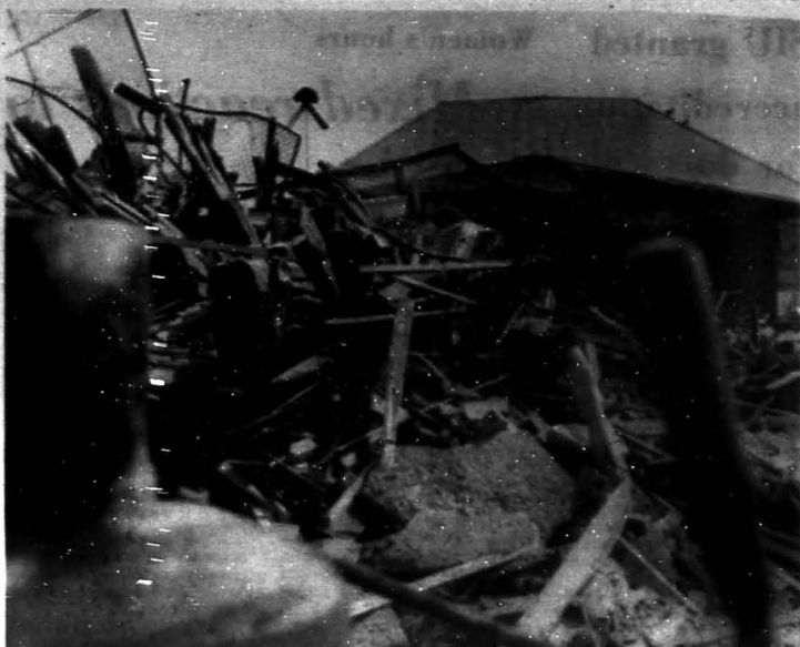
This is progress. The north section of the Illinois Central Railroad station in Carbondale was torn down Tuesday. The rubble will be cleared away sometime today and the property may be used as a bus turn-around area in the future. (Photo by Mike Ryan)
