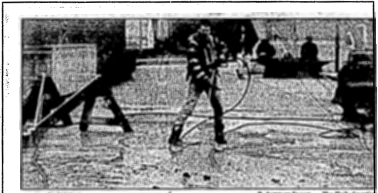
Mr. Clean: Kevin Snyder, an SIUC laborer, uses a high pressure spray Wednesday afternoon to clean up the sidewalk after his crew repaired a water line break at Life Science II.
