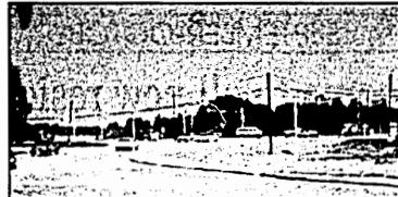
Another very visible project has been reconstruction of the intersection of Emerald Lane with Main Street. The project has been underway all summer and was just recently completed and reopened to two way traffic. The patience of the motoring public with the project is appreciated. Keeping one way traffic south-bound facilitated access to the businesses, but it also stretched out the construction schedule a few weeks. This project resulted in the creation of a left turn lane which will greatly improve the flow of traffic in this area.
