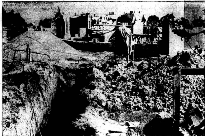
BATH HOUSE As this picture shows construction on the new bath house at Thompson Point Lake is well underway. When completed the bath house will be for the use of both students and faculty. It is hoped that it will be finished by next summer.
