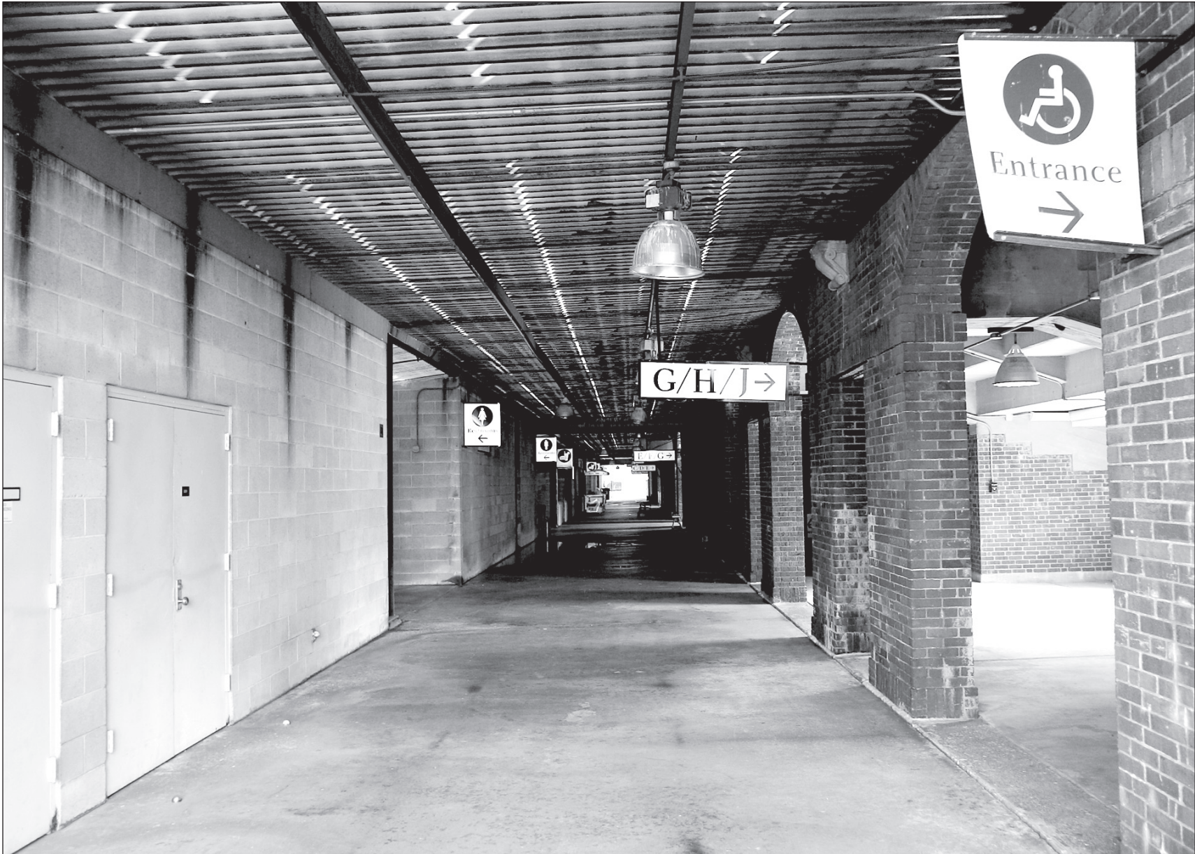
Water puddles from an early morning rainfall coat the floors of McAndrew Stadium's concourse. The floors, which are power-washed regularly, are stained from frequent leakage and water damage.
