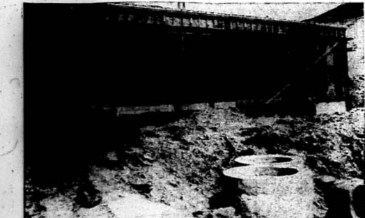
IN SUMMER This shot of a section of the new Home Economics Building was made back in July. At that time the frame for this section—which will be the Nursery—had just been completed. Construction during the summer months went on at a rapid rate and the new building is taking form.
