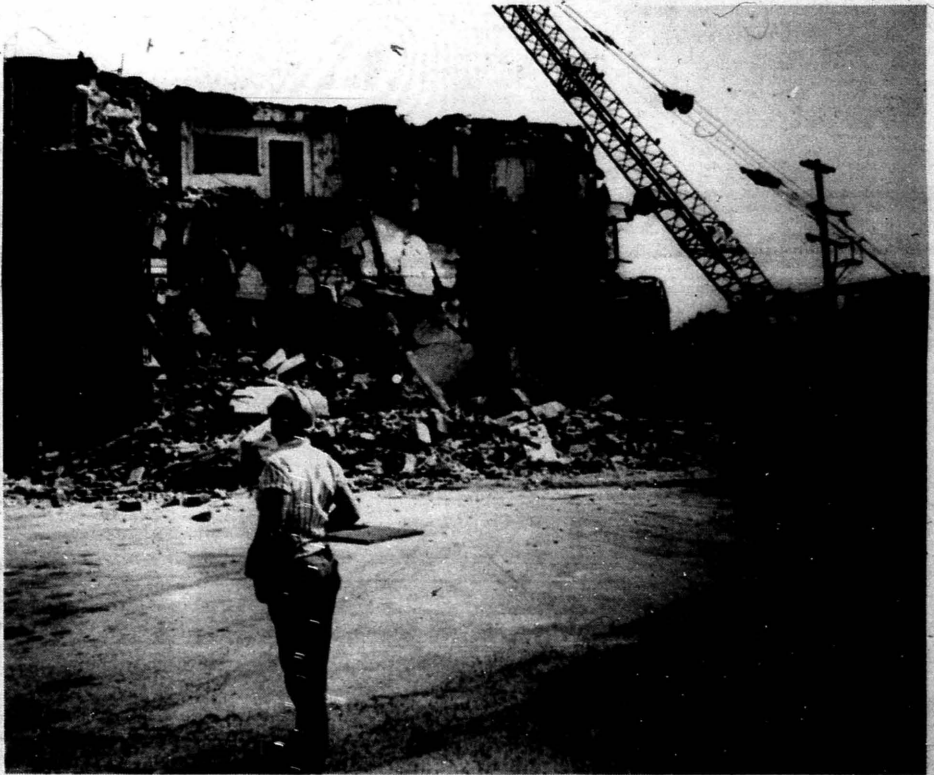
A workman watches as progress takes its toll on the vacant Holden Hospital building located on South Illinois Avenue. The demolition of the structure, which has been vacant for
