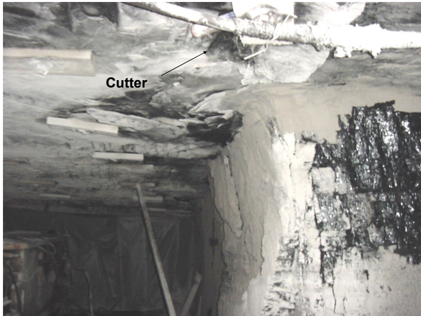
Photo 1: The onset of a cutter into the roof against the pillar rib
