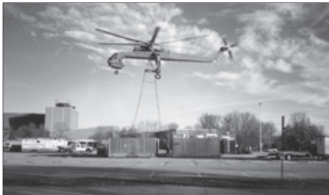
Olga lifts Marley, part of the cooling towers, for the final half-mile trip to the top of Morris.
