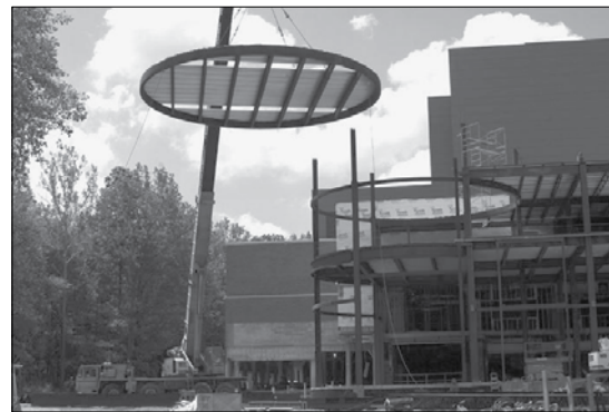
The installation of the roof of the rotunda, part of the new look of the north face of the Library, marked the halfway point in the major renovation of Morris Library.
