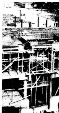
PROGRESS ON SIU's new library near fundamental structural completion as workers lay the building's roof. The library is expected to be ready for
