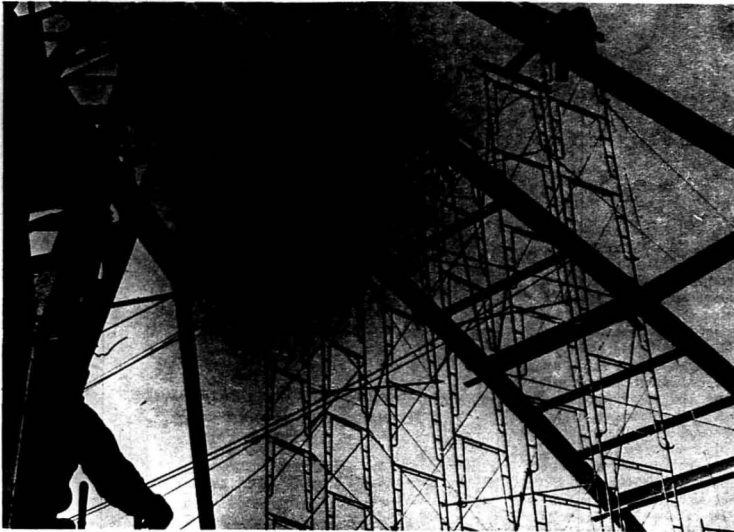
SIGN OF PROGRESS -- While students and faculty were away over the holidays, construction workers began putting into place the arched beams that will support the top of the dome of
